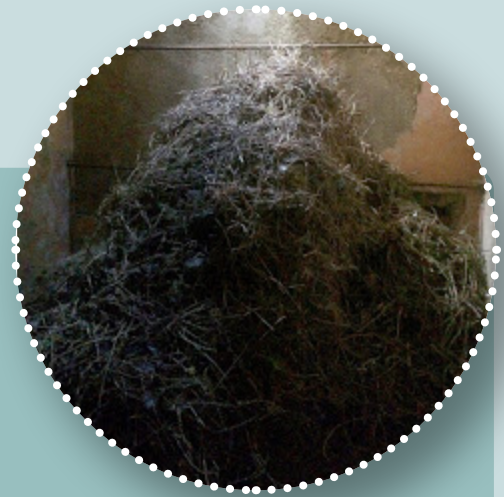
Jackdaw nest material has blocked the chimney of an abandoned farmhouse and has gathered at the fireplace
