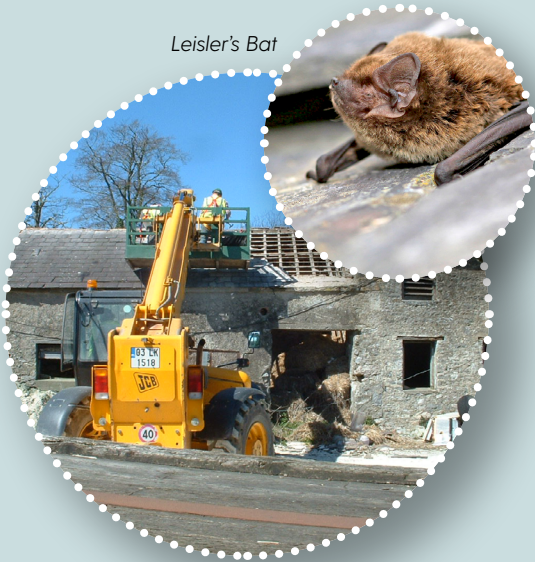
Careful removal of slates will ensure hibernating bats are discovered, and disturbance is minimised
